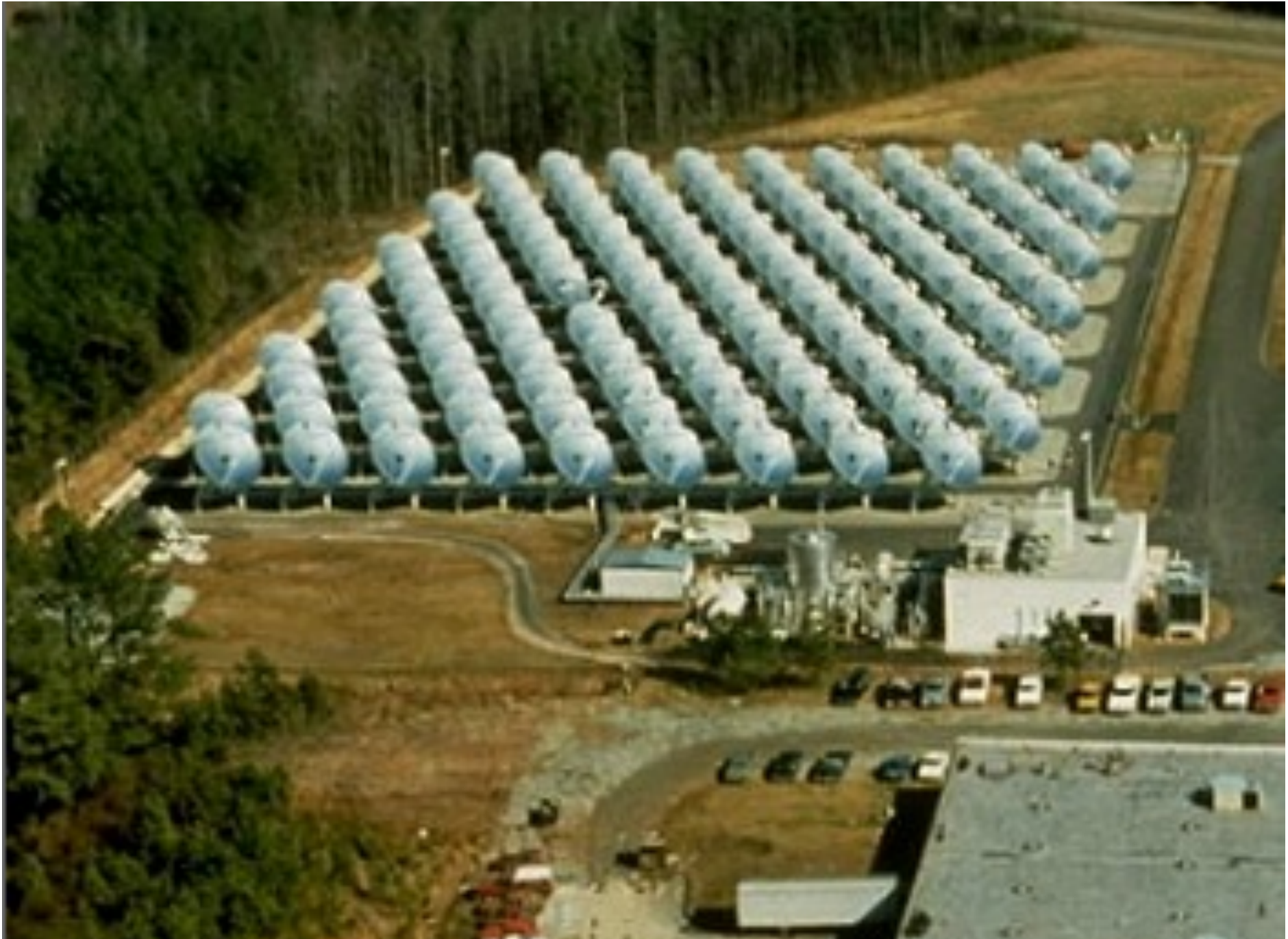
An array of 114 solar concentrators dishes
